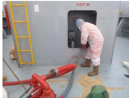
Wilden pump at F.O no. 3 vent
