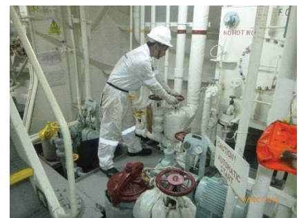
Opening VALVE for F.O transfer
